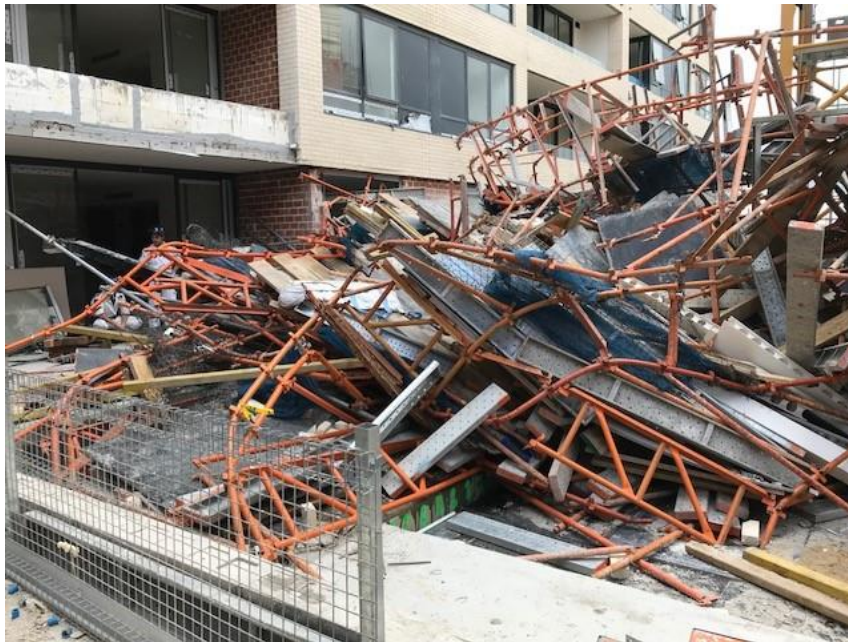
Image: Collapsed scaffold on the construction site where work was being done.
